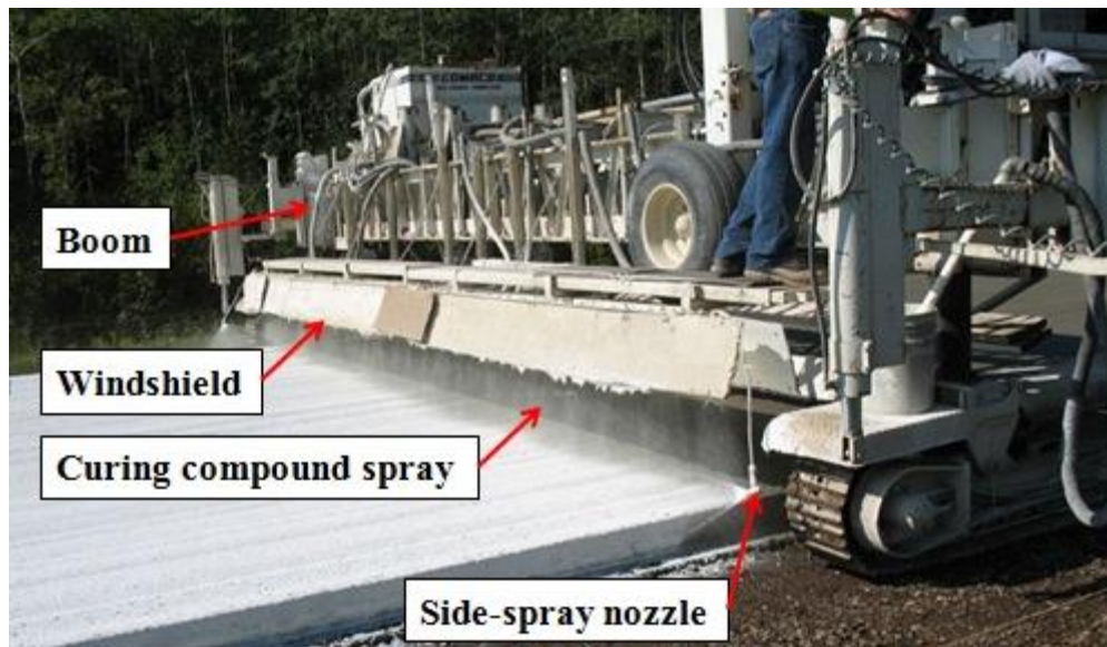
Figure 2.4. Spraying of curing compound using a paver machine (adapted from: “Poly-Alphamethylstyrene Concrete Curing Compound”, 2016)
